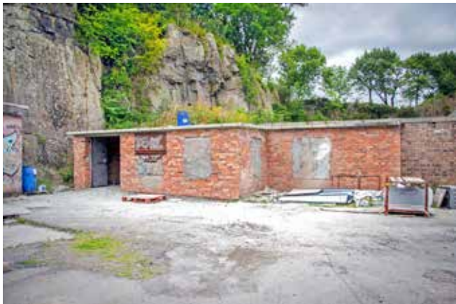
Front of the guardhouse looking good after a first pass with the media blaster. We have new windows ready to fit to the building
